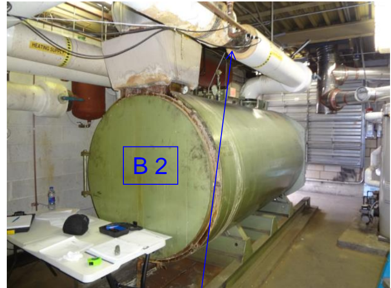
Boiler 2 Installed Flow Meter
