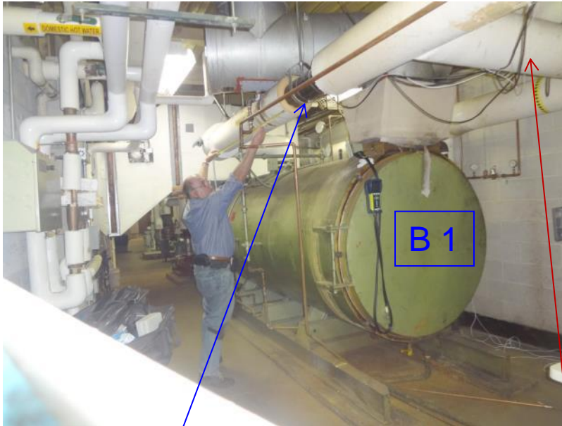
Boiler 1 Installed Flow Meter
